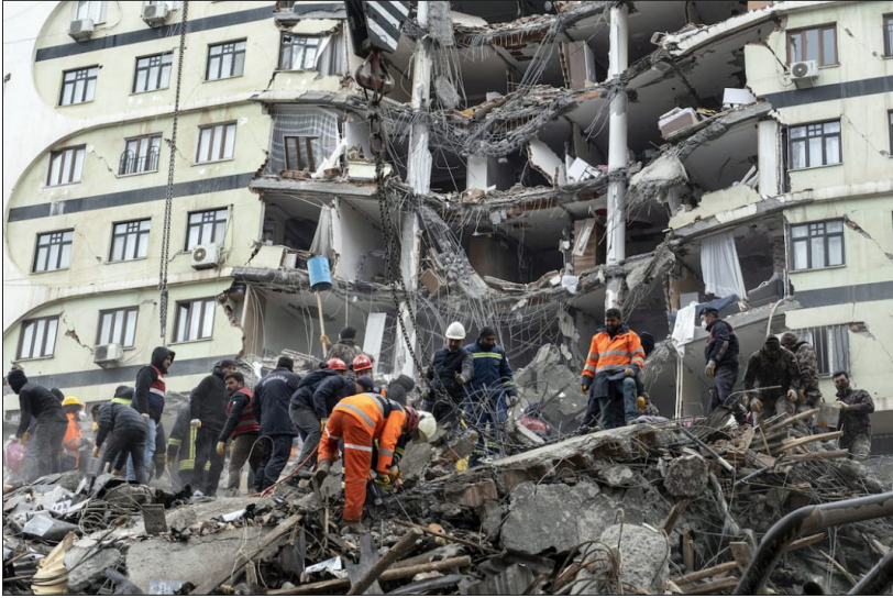
Figure 5. Destroyed building in Diyarbakir, Türkiye 19)
